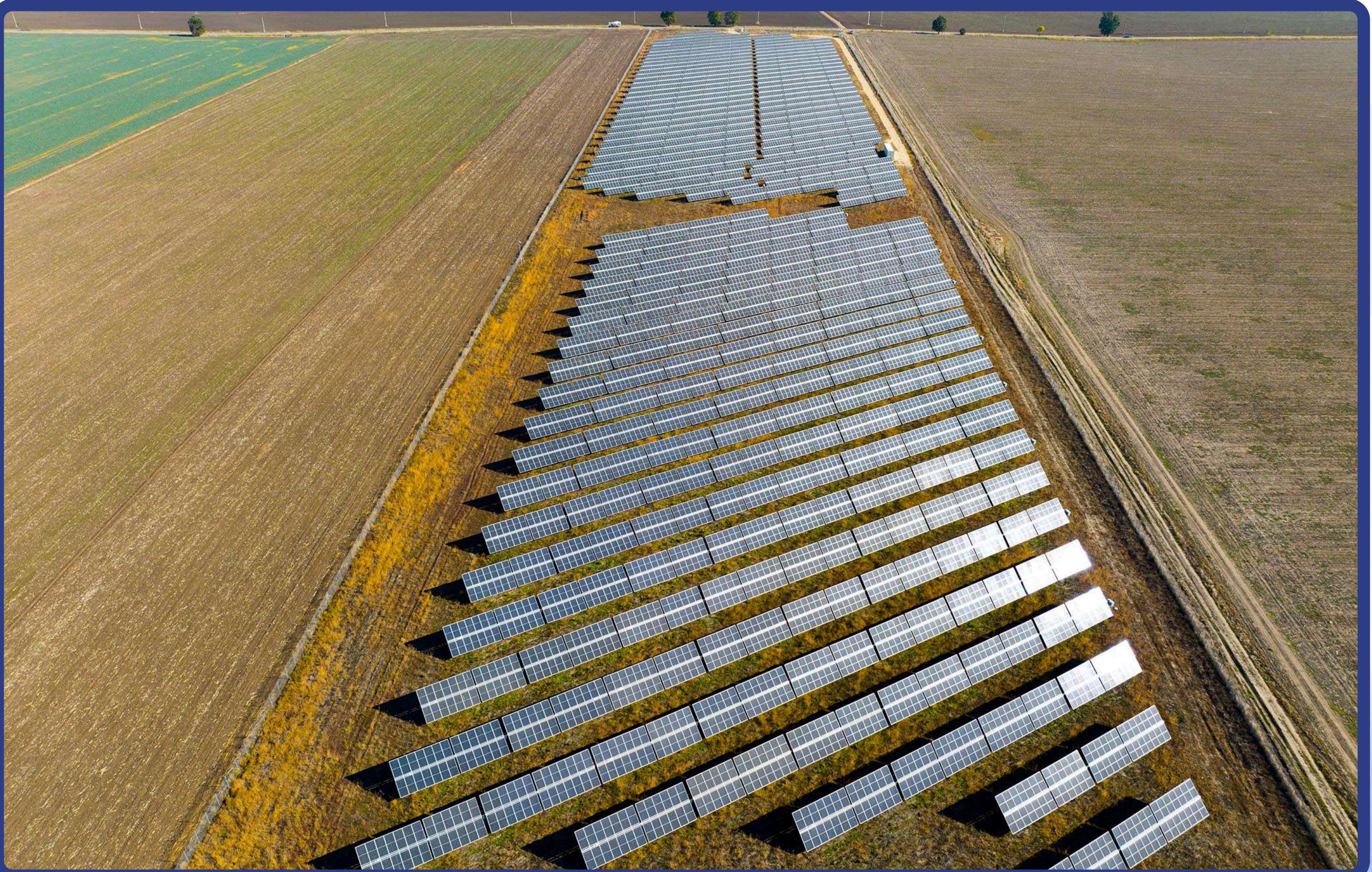
Alerion Italia- Rosiorii de Vede 5 MWp Valmont 2P tracker structure - Sep 2021 - Feb 2022
